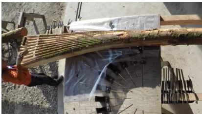
Spacers are placed between the layers of the 25cm diameter sliced log in preparation for steam bending. Image Credits: Design + Make, Sawmill Shelter
