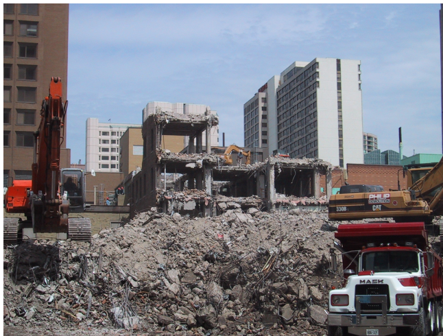
Figure 5. Demolition is more often the outcome of obsolescence rather than physical deterioration.
