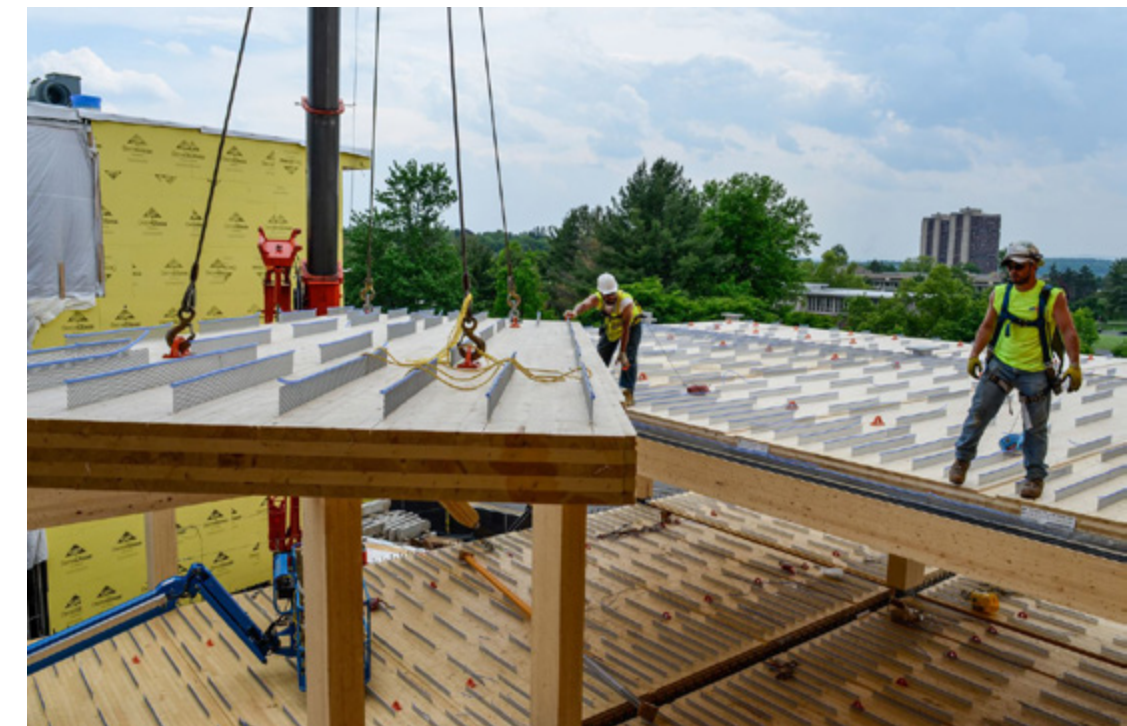
The efficient delivery and rigging (hoisting) of mass timber components is critical to gain the mass timber advantage. Efficient deployment of cranes and booms is an important erection strategy to optimize during the planning stage of a mass timber project. (Alex Schreyer/UMASS)
