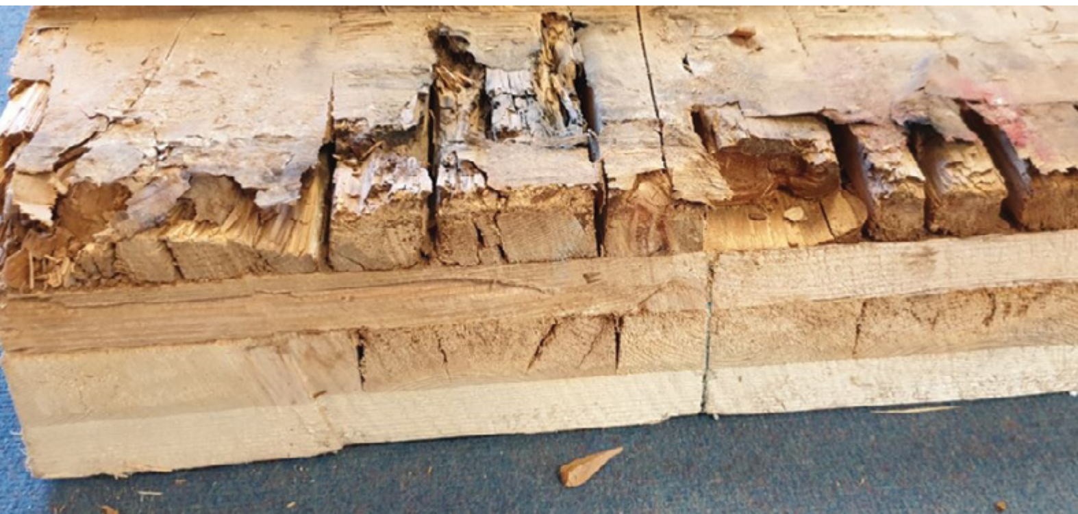
Exceeding the moisture balance of mass timber must be avoided. Moisture absorption for mass timber elements is a delayed process, however, it must be recognized that long-term or frequently recurring exposure to moisture is likely to be more problematic than the overall quantity of water to which the mass timber is exposed. This is because wood absorbs water rapidly and after it is saturated it releases this moisture very slowly as it dries out. In practical terms, trapped and concealed moisture must be avoided by providing multiple layers of defence against moisture intrusion. If the risk of moisture penetration cannot be avoided, then the assembly must be designed so that it is much easier for the water to get out than to get in. The severe deterioration depicted in the lower image occurred in a cantilevered CLT balcony panel suffering concealed moisture migration.
