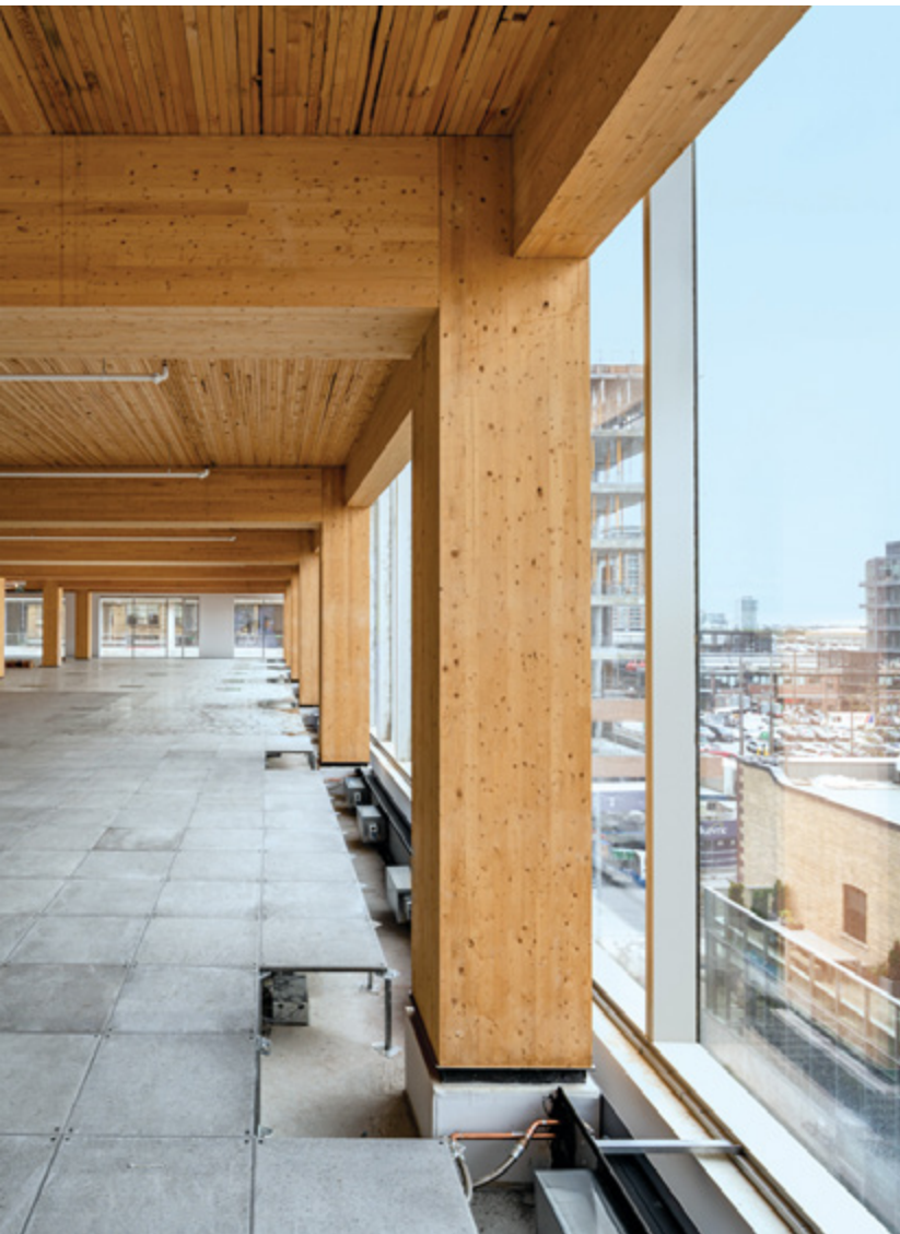
Raised floor systems help address acoustical issues. In addition to helping integrate mechanical, electrical and plumbing systems unobtrusively, raised floor systems, such as this one installed at 80 Atlantic, designed by Quadrangle Architects, also minimize the transmission of airborne and impact sound transmission across floor assemblies. Note that a concrete topping over the NLT floor panels is required to fireproof concealed cavities. (Bob Gundu, Canadian Architect)
