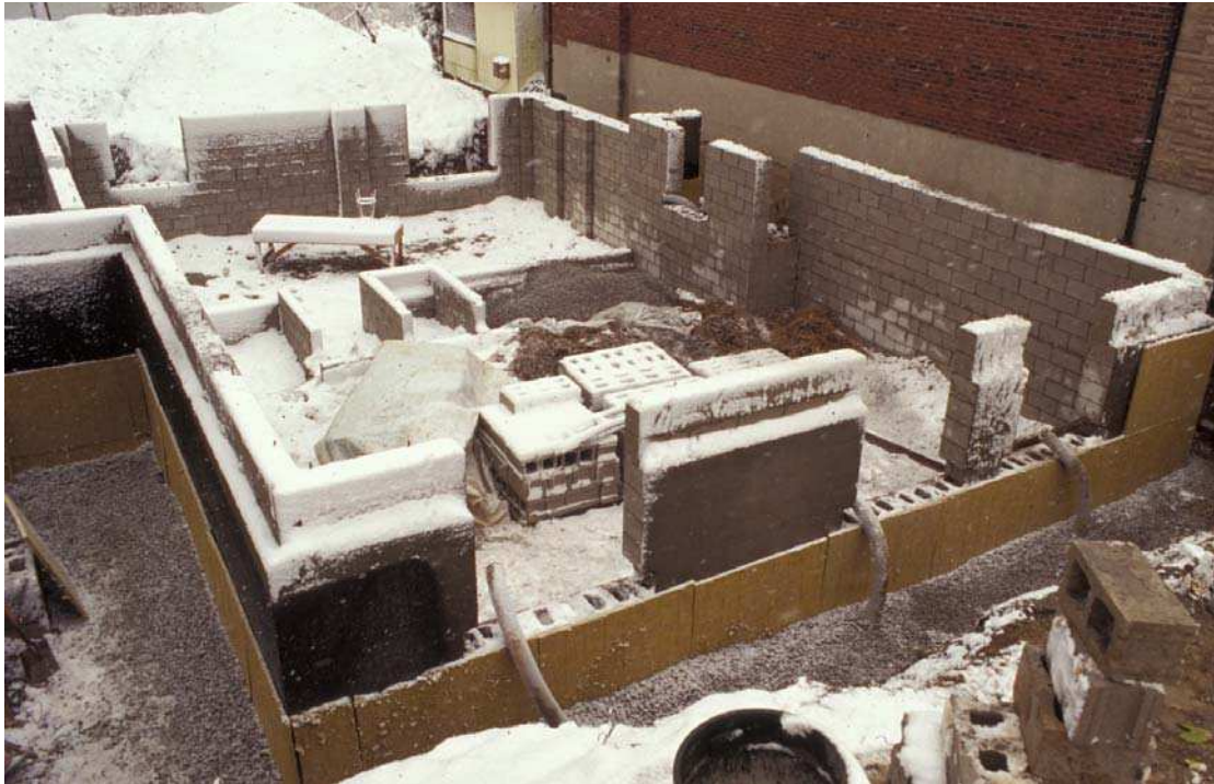
Figure 1.4 An example of construction moisture accumulation during winter construction.
