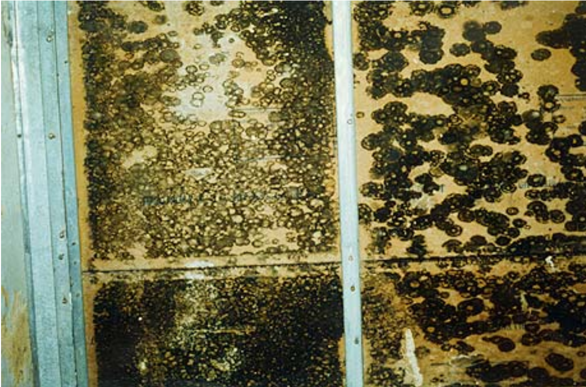
Figure 2. Heavy growth of S. chartarum and some other fungi on gypsum wall board in a flooded school basement. This growth occurred about one week after the flood. It was removed before remodeling. Source: Professor Berlin D. Nelson, Stachybotrys chartarum : The Toxic Indoor Mold, Nov. 2001. http://www.apsnet.org/online/feature/stachybotrys/
