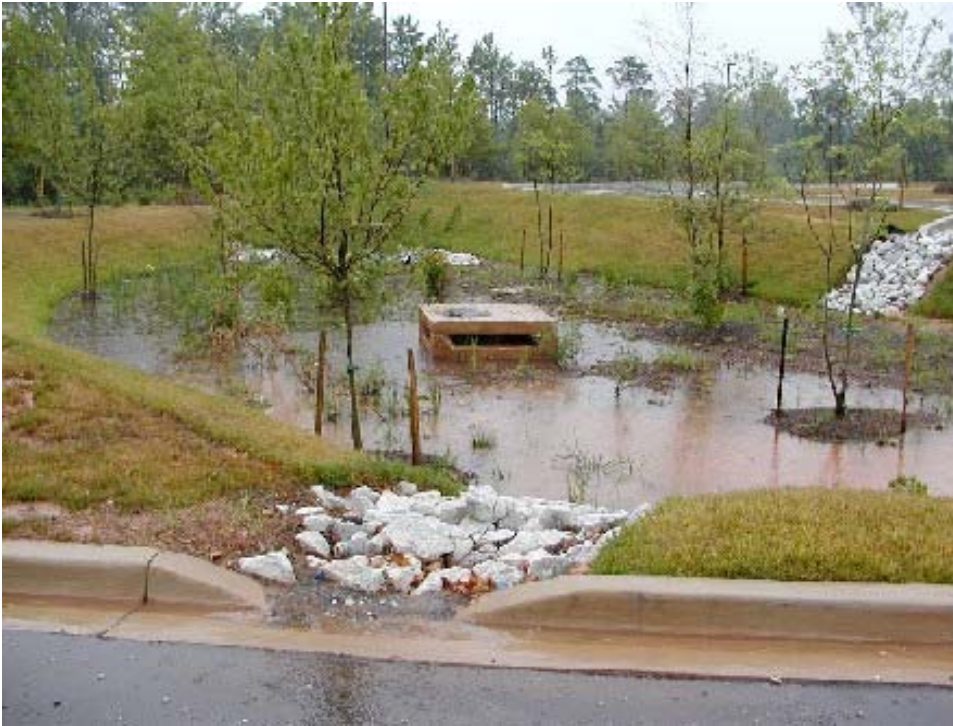
Figure 27. Rock rip-rap for erosion control is used at the inlets to the detention basin. Note the pre-cast concrete overflow control structure.
