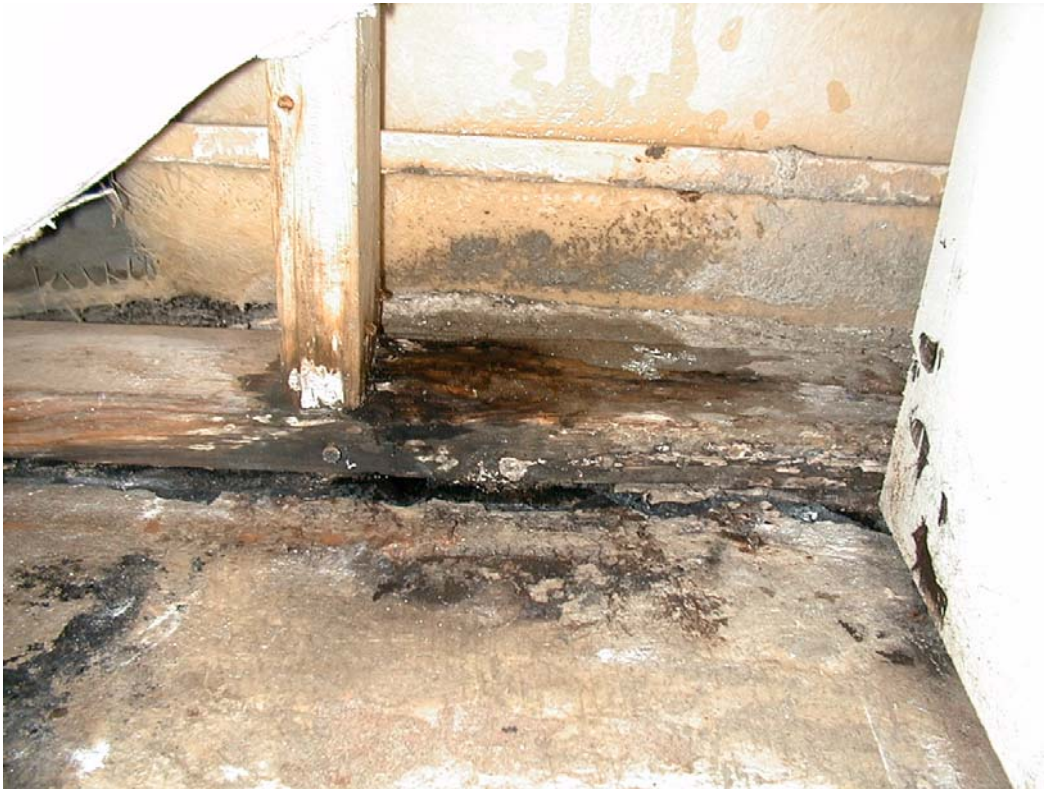
Figure 1. The effects of basement flooding, revealed above after removing a section of wall board, are often hidden by cosmetic repairs to interior finishes, leaving occupants susceptible to long term exposure to molds, often unaware of associated health risks.
