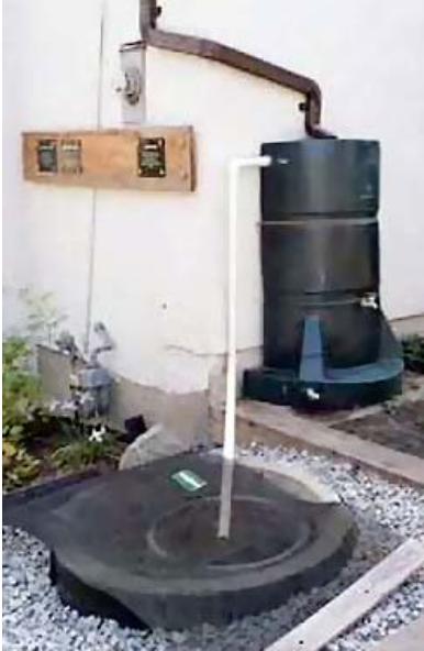
Figure 9. Downspout disconnected from municipal sewer system discharges to a rain barrel connected to a soak pit. Savings in potable water use for irrigation along with reductions in pollution and sewage treatment costs are benefits that extend beyond basement flooding protection.
