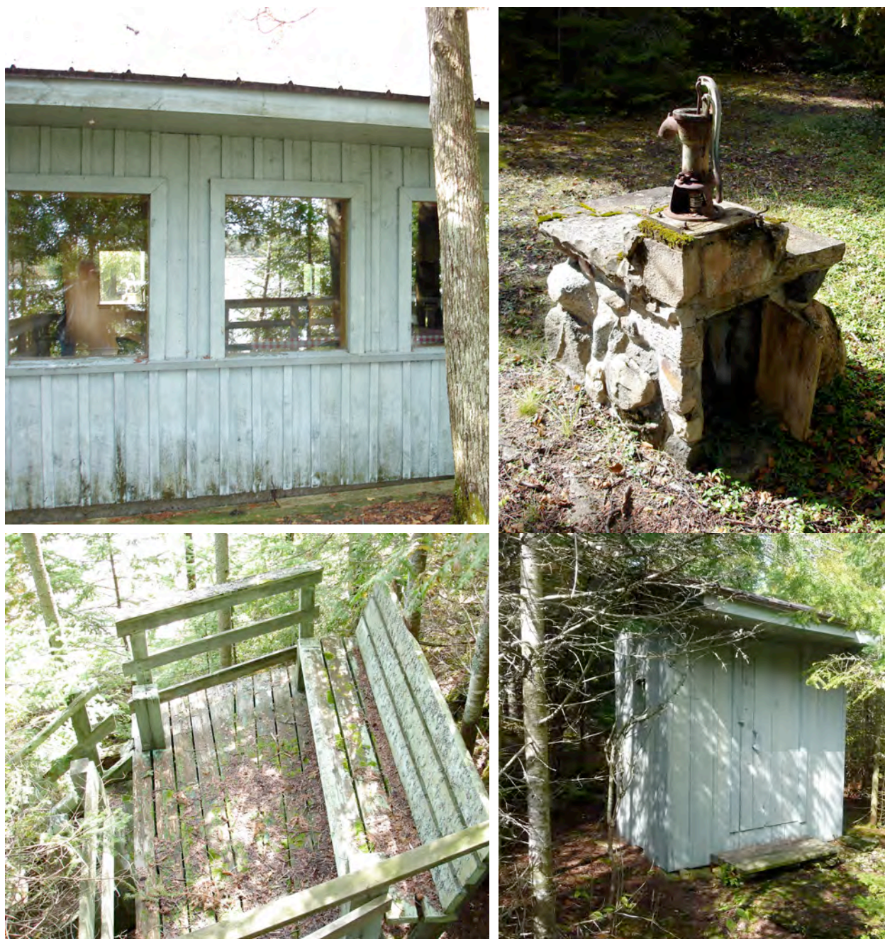
Figure 10. Deterioration of the wood siding is evident on the east elevation (top right), The well was reported to be functional, but the hand pump is in a state of disrepair (top right). 9 The questionable condition of an observation deck has caused it to be barricaded from visitors (bottom left). The privy building is in good condition, but no longer permitted for use by environmental regulations governing Ontario parks (bottom right). 2010.
