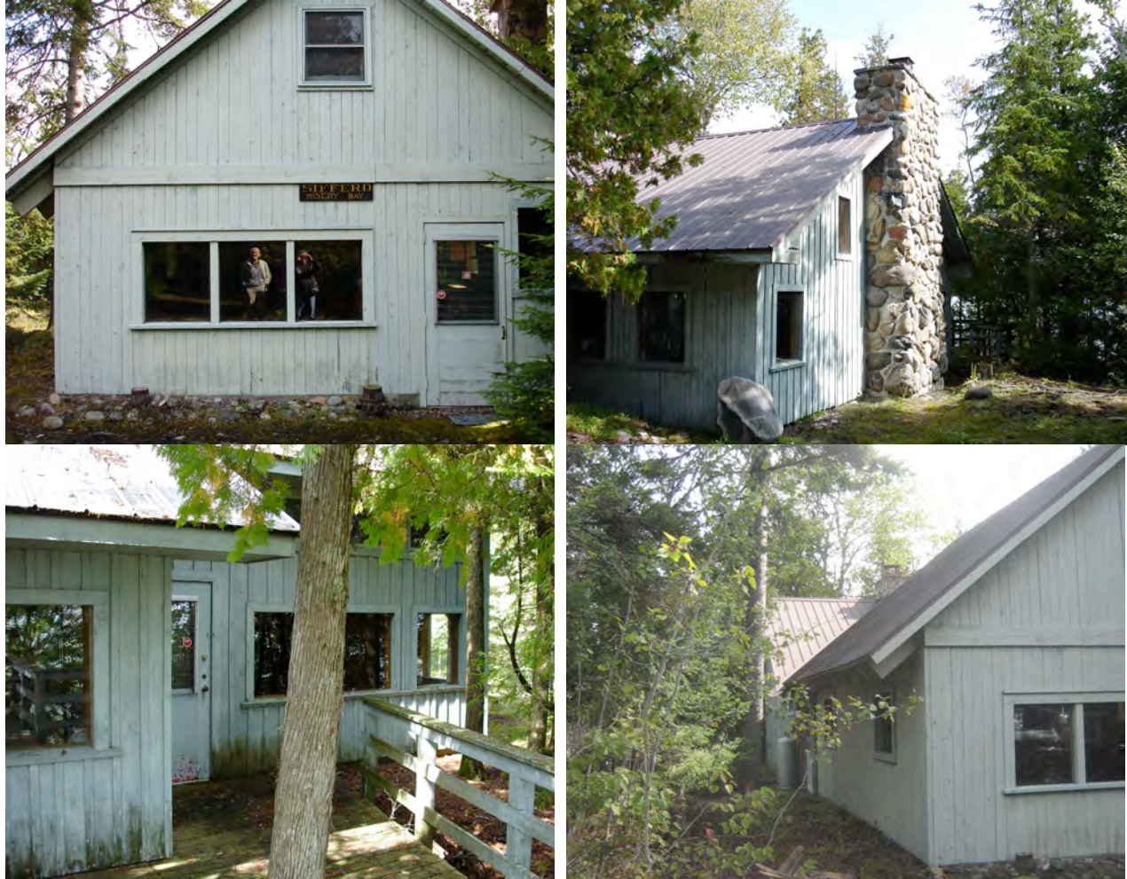
Figure 9. North elevation of Sifferd Cottage (top left). The South elevation features a massive stone fireplace. (top right). Accumulations of leaves and twigs near bottom of siding allowed to remain without routine cleaning have initiated deterioration of the wood siding (bottom left). The roof structure is straight and true, and the metal roofing is in good condition, but some of the chimney flashings require repair and/or replacement (bottom right). 2010.
