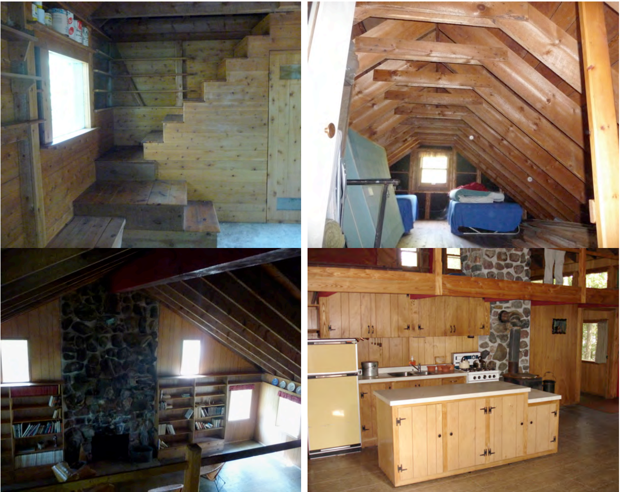
Figure 11. Railings for stairs leading to upper level are missing (top left) and railings for stairs leading to mezzanine, as well as mezzanine guards (bottom left and right) do not comply with Code requirements. Attic loft must be cleared of clutter to afford safe egress (top right). 2010.
