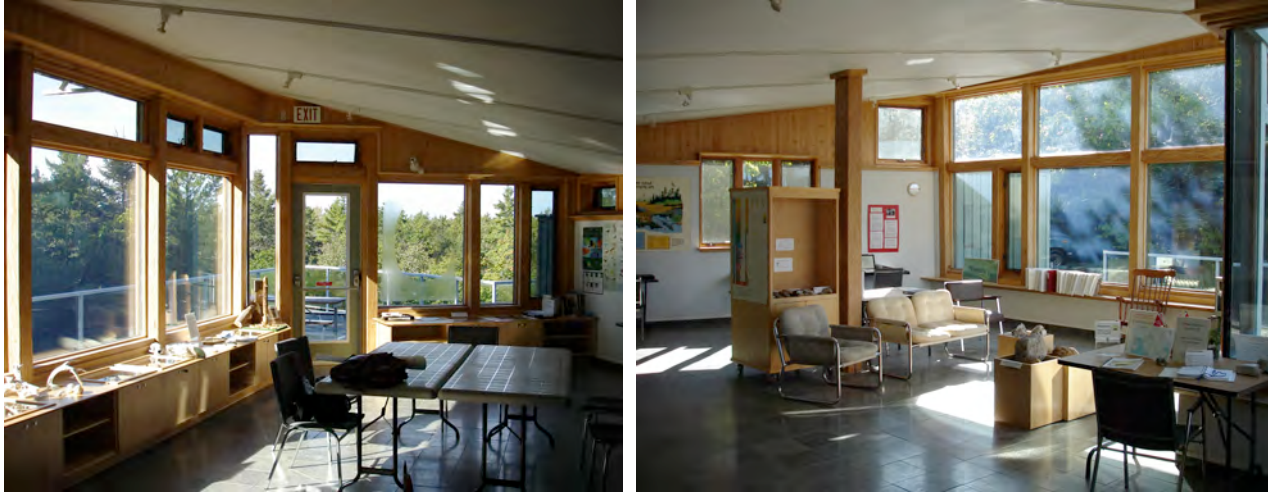
Figure 5. Interior views of the Visitors Centre indicate a clean and dry facility with all finishes and furnishings in good order. 2010.
