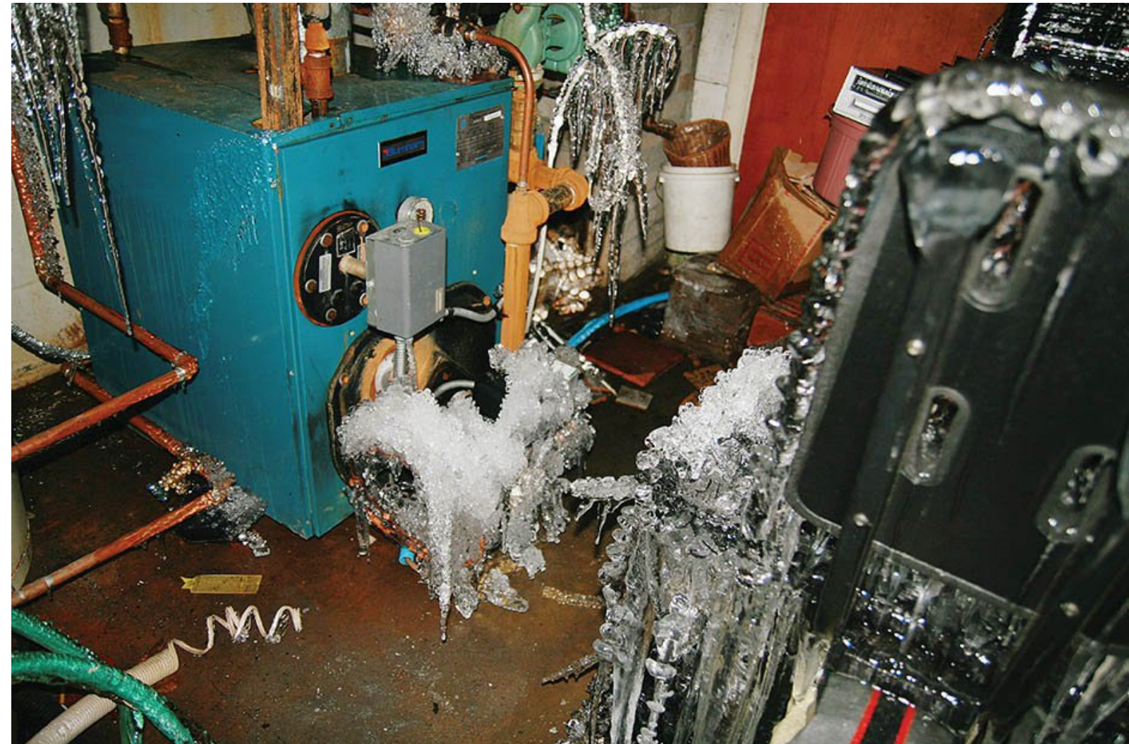
Thermal resilience modelling is imperfect, but still very useful. Predictions about how long it takes pipes to freeze after a power failure in winter are imprecise, but the risks associated with various levels of thermal control can be comparatively assessed to inform prudent preventive measures. [Photo courtesy Insurance Adjusters Canada Inc.]
