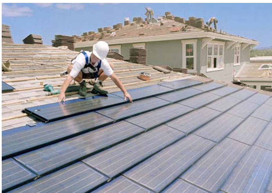
Figure 30. Innovative PV technologies integrate energy collection with functional elements such as roof cladding. [Photo courtesy CMHC.]
