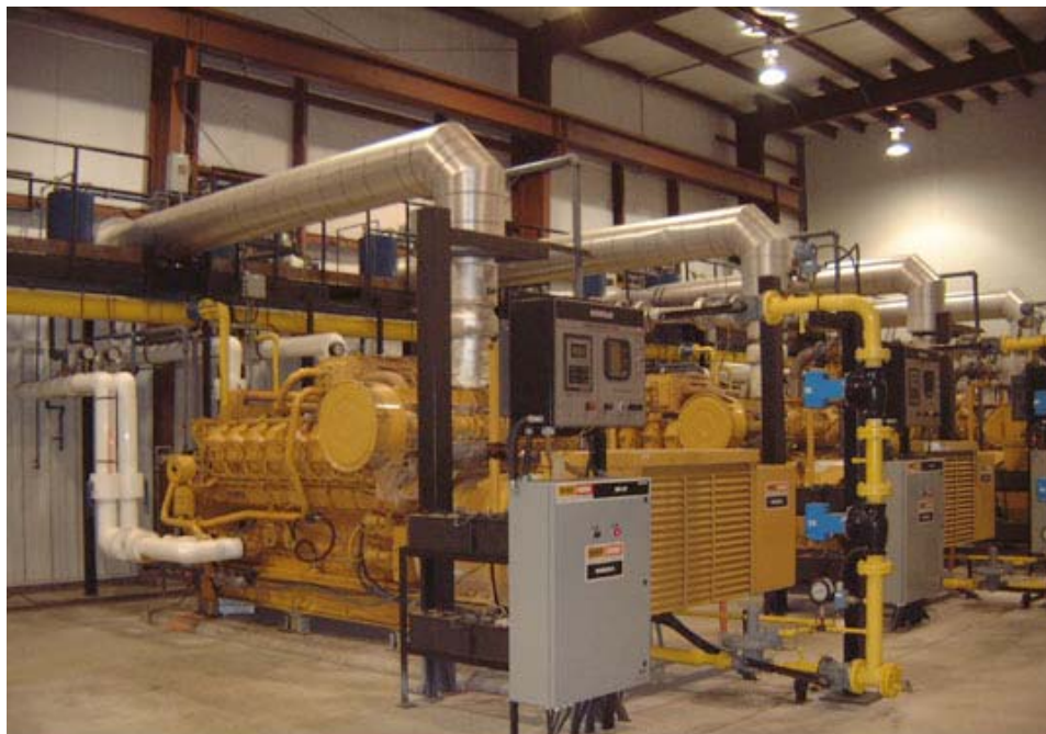
Figure 42. Converting landfill gas to electricity reduces greenhouse gas emissions and conserves non-renewable energy resources. [Photo courtesy City of Ontario, California.]
