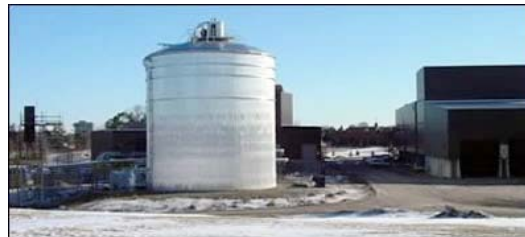
Figure 43. Anaerobic digester at Dufferin Organic Processing Facility, North York. [Photo courtesy City of Toronto]
