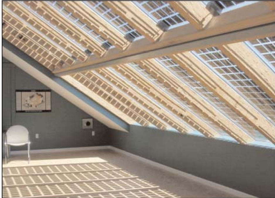
Figure 31. Thin film PV technologies integrated into glazing can provide both energy collection and environmental separation. [Photo courtesy CMHC]
