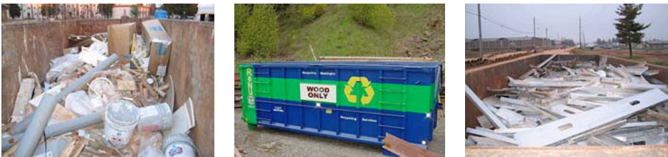
Figure 24. Construction waste management practices range from none (left image) to properly managed recycling facilities (centre and right images).
