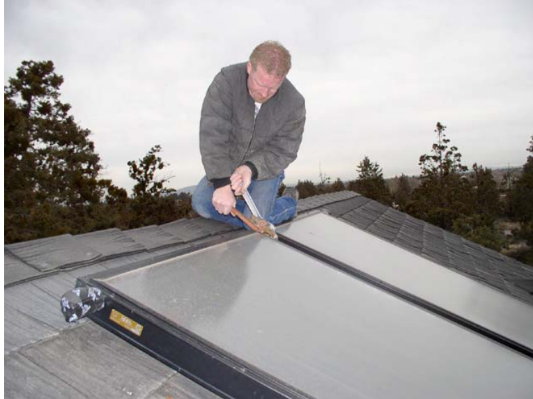
Figure 29. Solar water heater technology is less complicated than in-floor hydronic heating systems and can be reliably installed by plumbing and heating trades.
