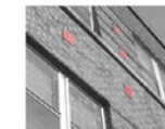
1. Original brick temporarily tied back to wood structure with steel plates before commencing renovation
