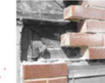
2. Destructive testing to assess condition of bricks and steel lintel and dryness of wall assembly
