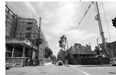
Construction of Six Four Nine Lofts also began on Flor 401 Lofts at 7 & Wall and SP7 at 7th & San Julian. In total there are currently 254 homes in construction on 7th Street, and more in the pipeline for Los Angeles and beyond.
