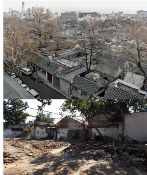
Demolition of courtyard houses in XianYuKou as part of the "Weigai" system for commercial development
