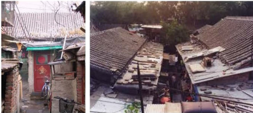
Courtyard open space is occupied by extension buildings, blocking sunlight. Lack of space: average living space per family (3.5 members): 15m 2 . China's official average: 20.23m 2 /person
