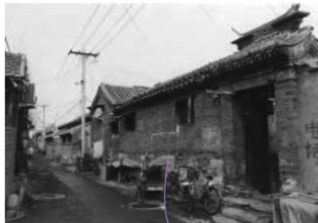
Deteriorating façade with minor repair
